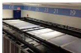
Full Cold Aisle Containment Utilized to contain air; panels shrink and fall under high heat
