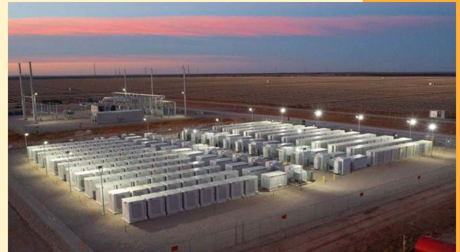
Azure Sky solar + storage, Haskell County (Texas) (Photo by Enel Green Power )
