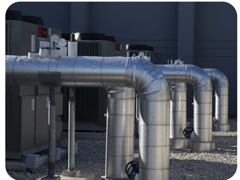
Dallas (DFW3) Water-free Cooling Equipment
